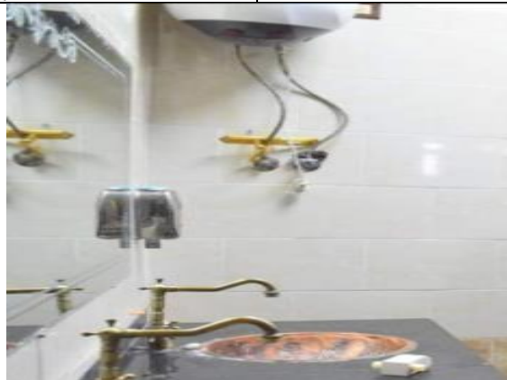
Example of automatic water taps (Beni-Suef University, Beni-Suef)
